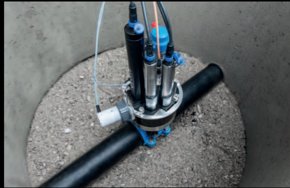
Example of an Installation in a Manhole
